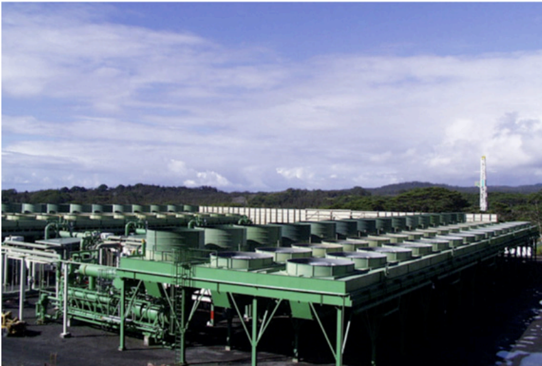
This power plant provides about 25% of the electricity used on the Big Island of Hawaii. It is a hybrid binary and flash plant.
